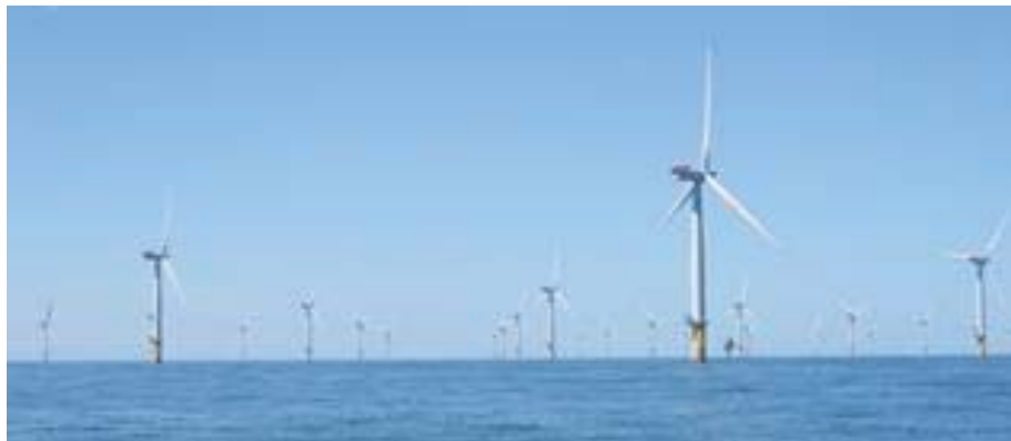
Sheringham Shoal Offshore Wind Farm, UK (317MW (3.6MW x 88)) (Photo by Yoichi Oda May 2014)
